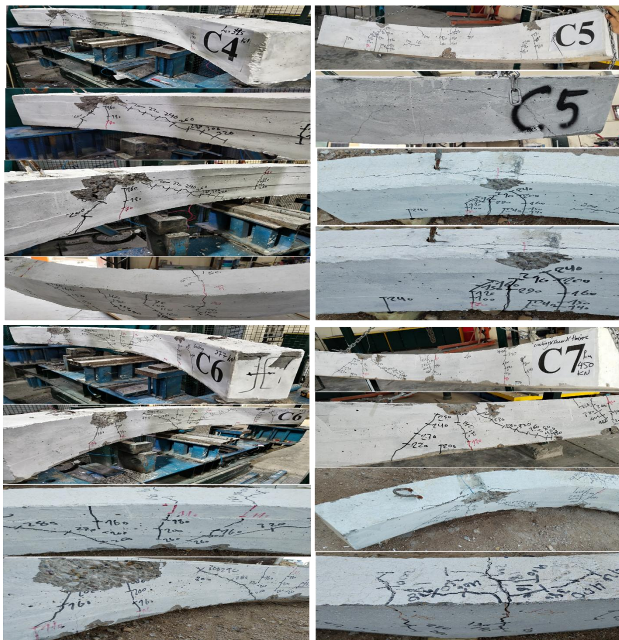
Figure 6 Modes of failure for tested beams
